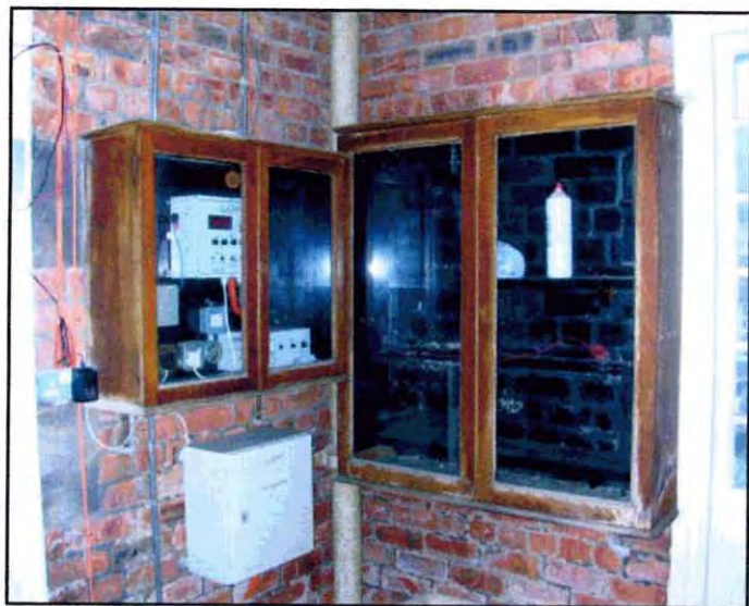
The cabinets that would have held the Batteries, right and the Charger, left.
